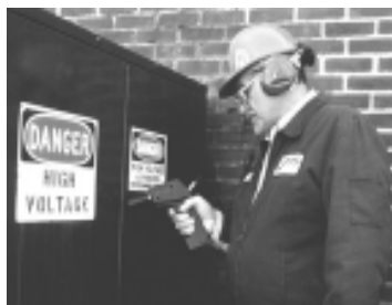
Test switchgear, transformers, etc. for arcing, tracking & corona.
